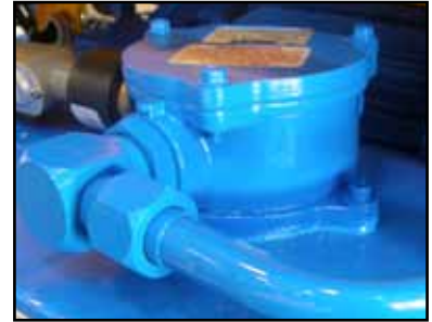
Figure 7-5: Return Line Filter
