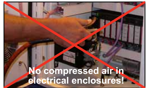
Figure A-1: Never Use Compressed Air Inside an Electrical Enclosure
